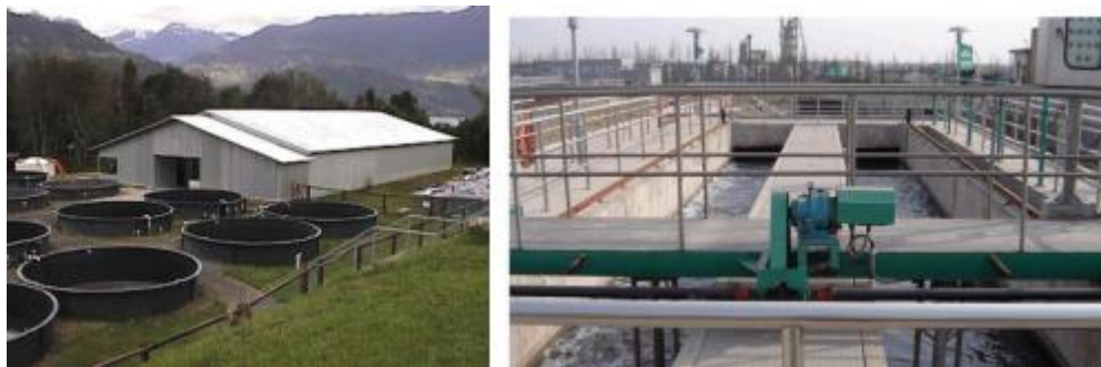
Figure 1: ATE1200 Application in Wastewater Treatment Plants
